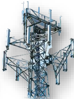
Antennas, Cellular Base Stations & Wireless
